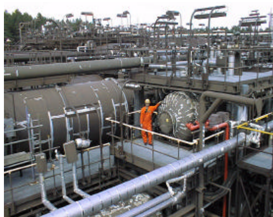
Figure 6. General view of the separator
